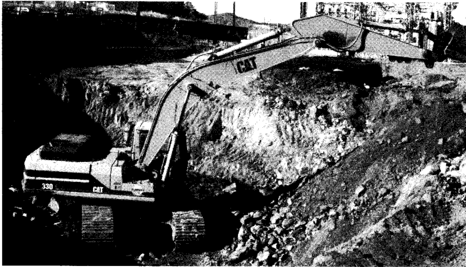
Approximately 60,000 tons of contaminated soil had been excavated by the end of June. The project is expected to be completed in about October.
