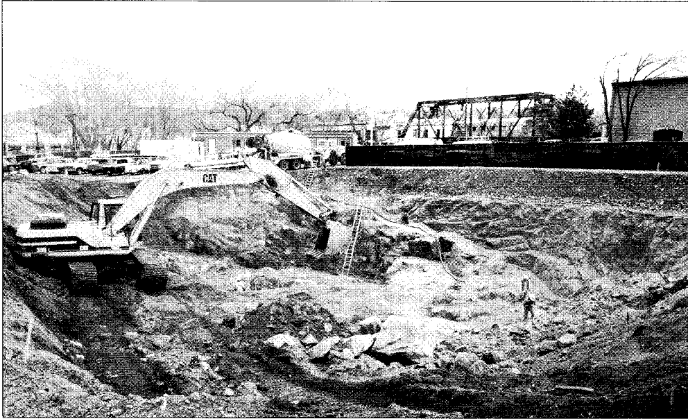
Excavation required skilled heavy equipment operators trained to work under stringent safety standards.
