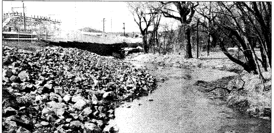
The creek flowing alongside the APS substation was protected throughout the contamination clean up project.
