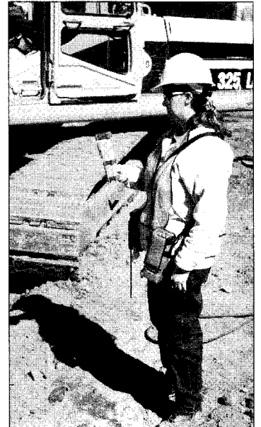
Air sampling was done continuously to ensure the safety of workers and residents.
