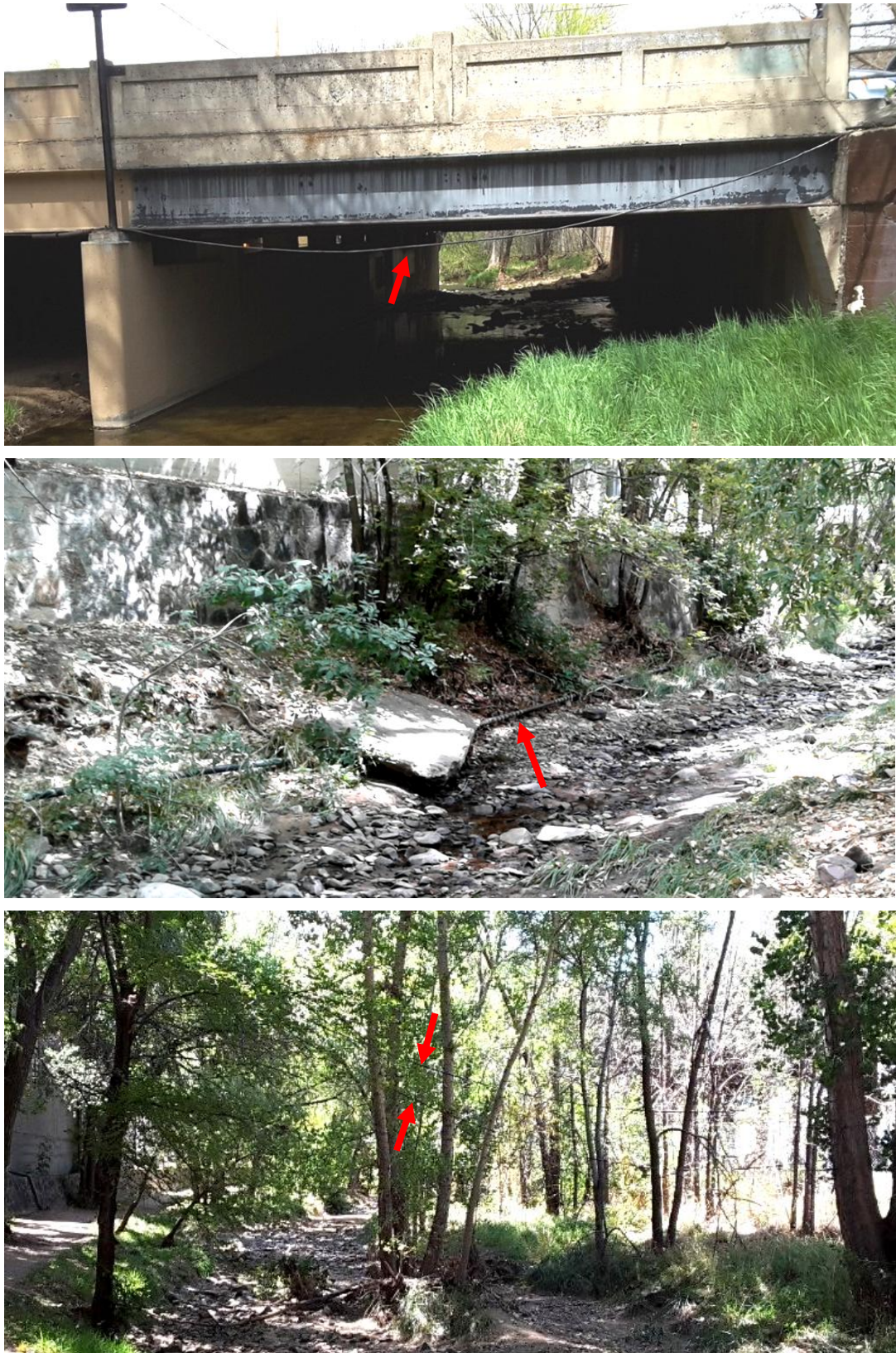
Figure 16. Utilities that may be in need of repair.
