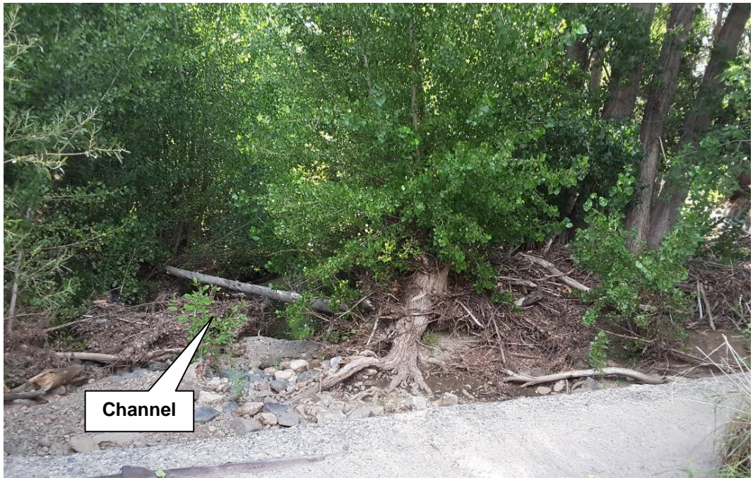
Figure 13. Dense vegetation blocking floodplain downstream of Carleton Street.
