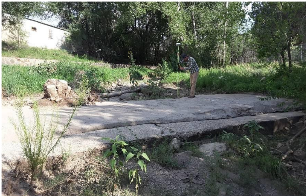
Figure 10. Utility crossing creates an overly wide, shallow cross section.
