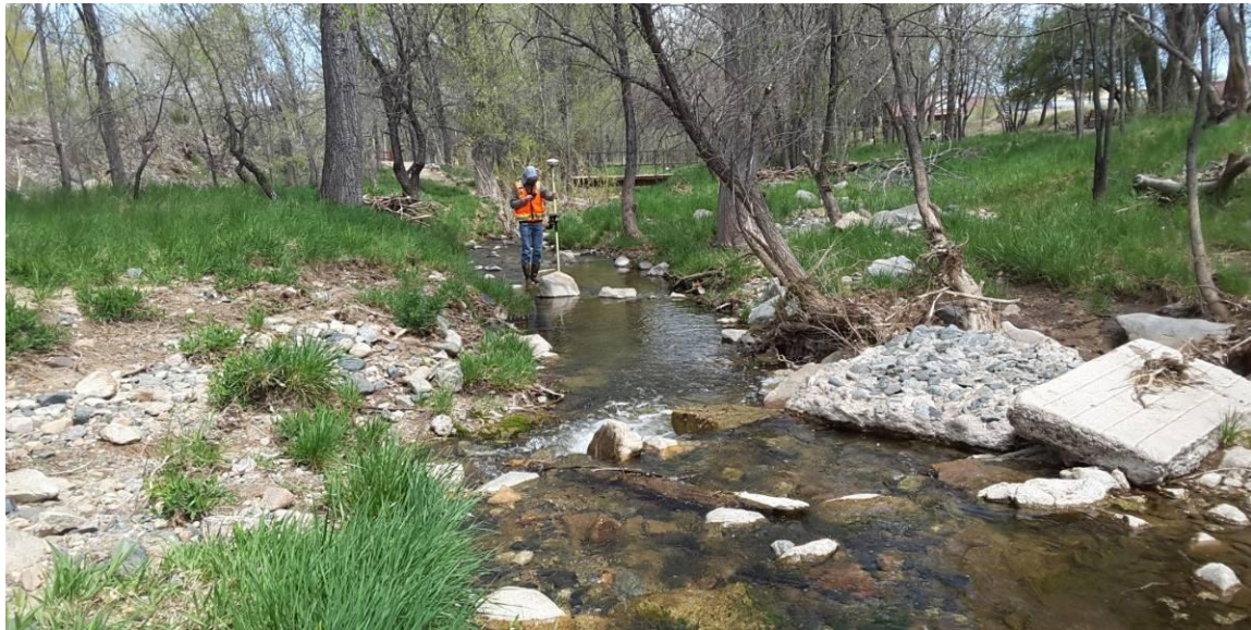
Figure 21. Concrete debris in channel.
