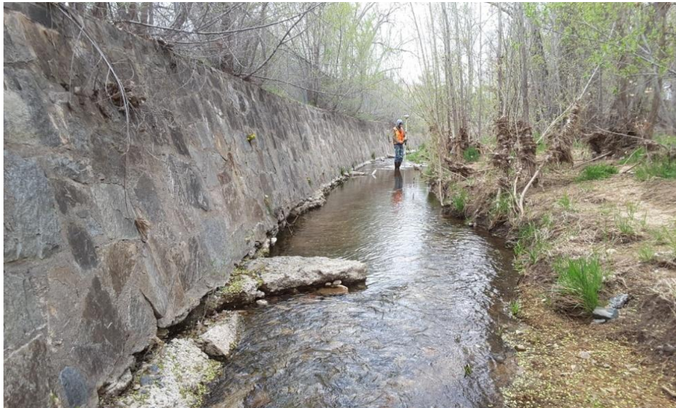
Figure 20. The foundation of the wall is being undermined.
