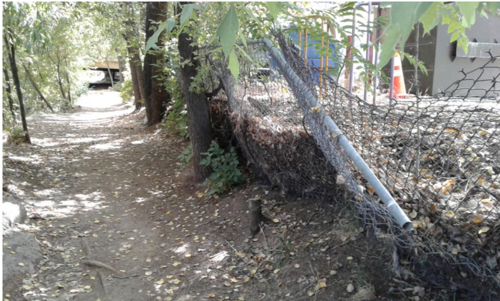
Figure 17. Two examples of fencing that are deteriorating.
