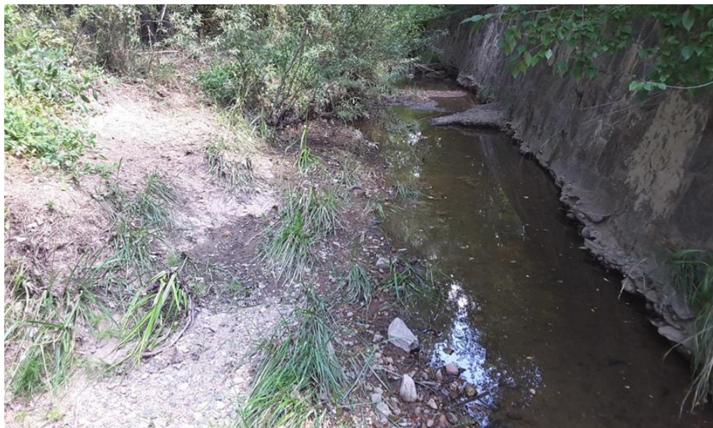
Figure 6. Bed scour undercutting retaining wall where floodplain is overly narrow.
