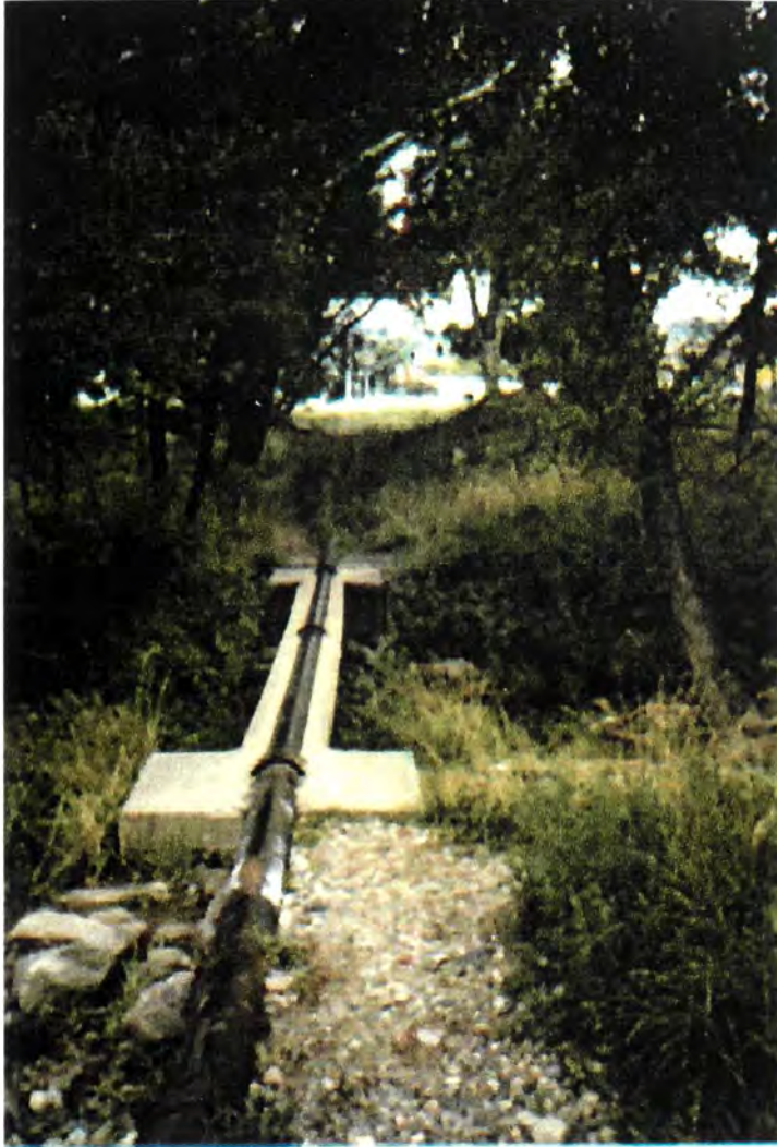
Current unsafe sewer line crossing being used to cross Granite Creek
